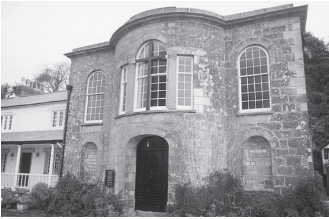
Figure 7. Pentewan Church. Note the repair on the right hand side, which has probably been carried out with an atypical Pentewan-type stone, which may not have come from Pentewan.
