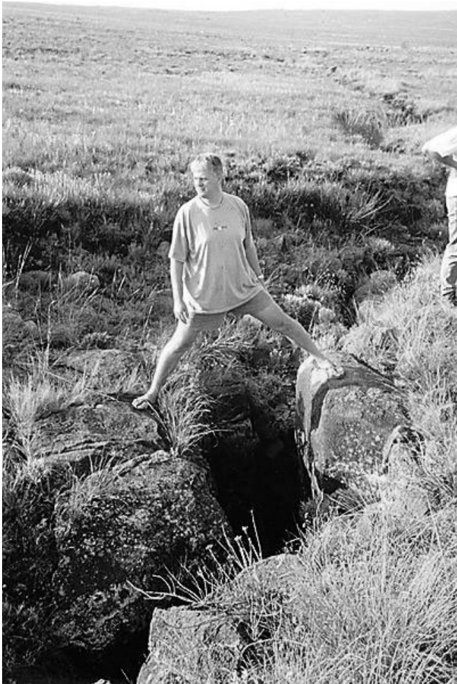
Figure 7. One of several major fractures in the summit plateau of Hlobane Mountain, KwaZulu-Natal, South Africa, caused by fracturing of a dolerite sill overlying superimposed underground workings in three coal seams (the Alfred, Gus and Dundas seams) worked from Hlobane Colliery. In this particular case, the large crack corresponds to the rib-edge of zones of total extraction in all three seams. William Pulles of PHD Inc bravely provides the scale.
