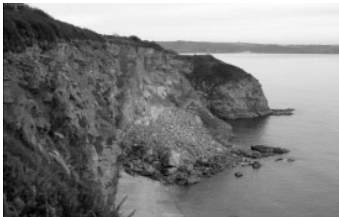
Figure 2. Wedge failure in the cliffs directly in front of the Carlyon Bay Hotel.
