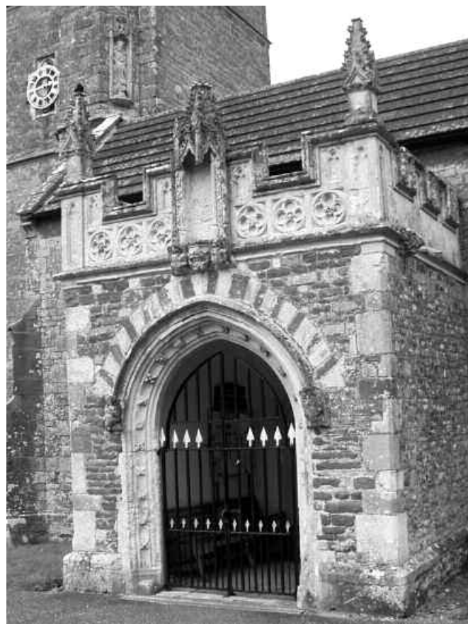
Figure 5. Porch of Talaton Church. Walls are predominantly of Bude Formation sandstone with minor chert and lava from the Exeter Volcanic Group. The quoins are of a mixture of Salcombe stone (Upper Greensand) and lava and the parapet and dressings round the door are of Beer Stone.
